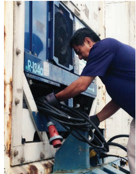
Okinawa DC's Yoshikatsu Ikemiyagi uses protective gloves while securing electrical cables to a unit.
